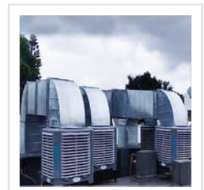
Industrial Evaporative Cooling System
