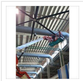
Industrial Factory Fabricated Ducting
