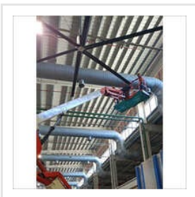
Industrial Factory Fabricated Ducting
