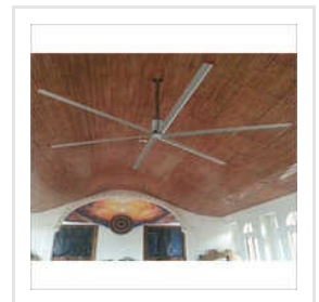
Industrial High Volume Low Speed Fan
